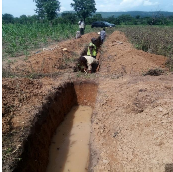
Fig. 19: Showing the Trench dug at point 4 to establish the extent of the quartz vein, here the vein was not seen and meaning the vein did not extend to this point or it is occurring as very great depth here. (N 9.170473734 o , E 6.912067875 o ).
