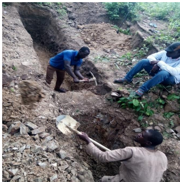
Fig. 13: 14 meters long Trench 1 was created perpendicular to the vein for sampling at the first contact point with the vein at the stream channel. (N 9.167856303 0 , E 6.911962193 0 )
